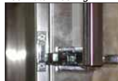
Door Latch Too Low
